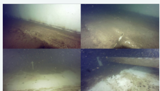
TANK FLOOR PLATES
